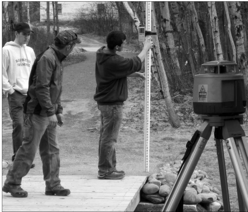
Clay Forrest and Gabe Winch use a laser to determine which corner of the bridge needs to be raised, as UTC instructor John Milligan looks on.
