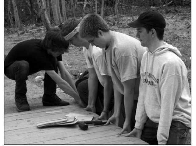
Not everything is high-tech. ACE students leveled the bridge by lifting it up, while one student inserted shims.
